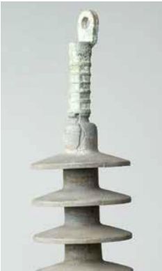
Sample damaged by erosion
