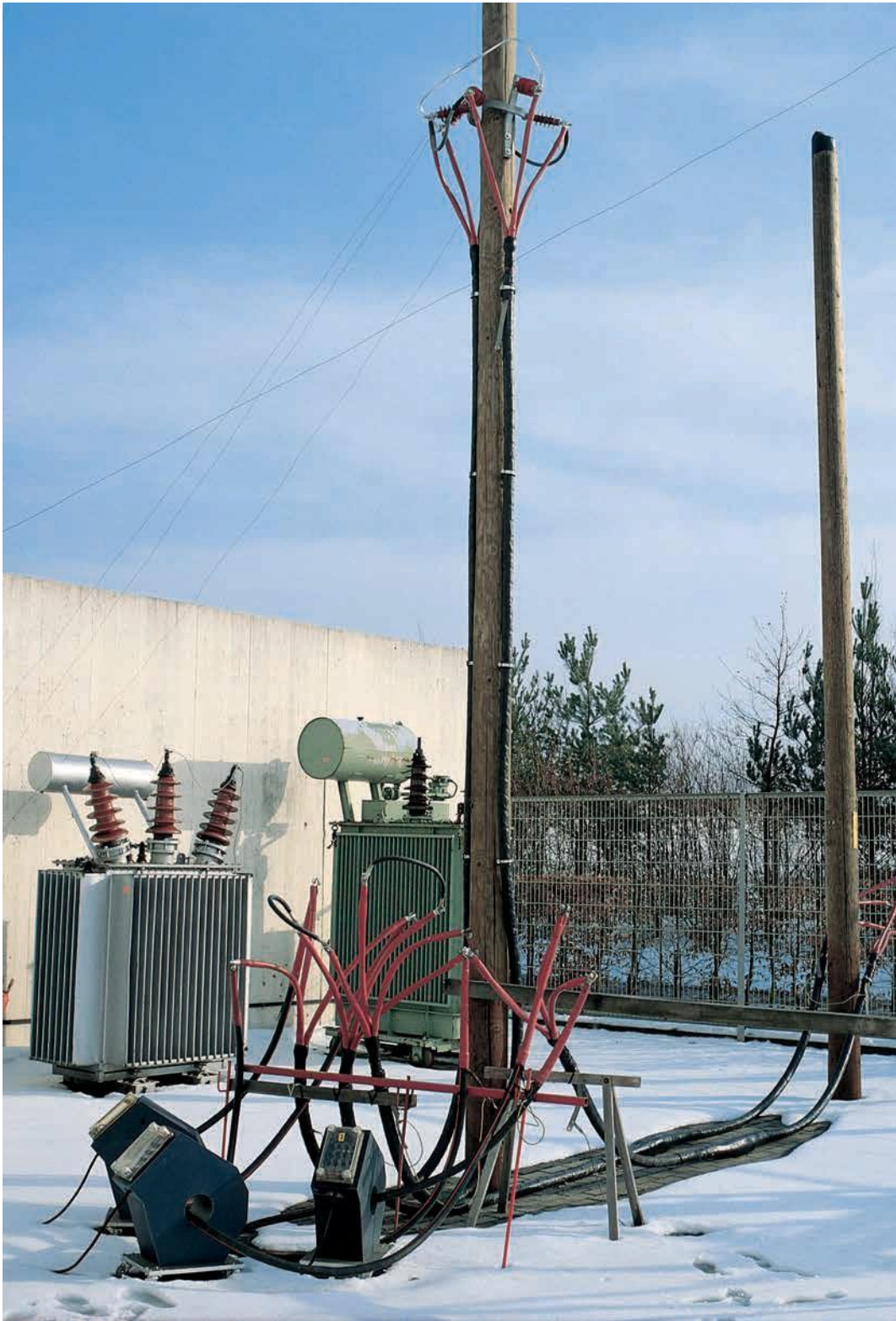
Long-term test of GUST-12 termination and GUSJ-12 joint on paper-insulated cables in the laboratories of TE Connectivity's research center.
